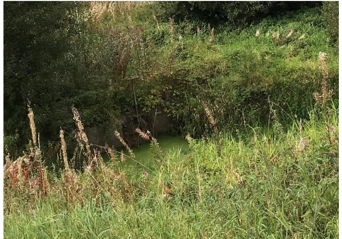
Sluice gate arrangement at diversion channel to pond
