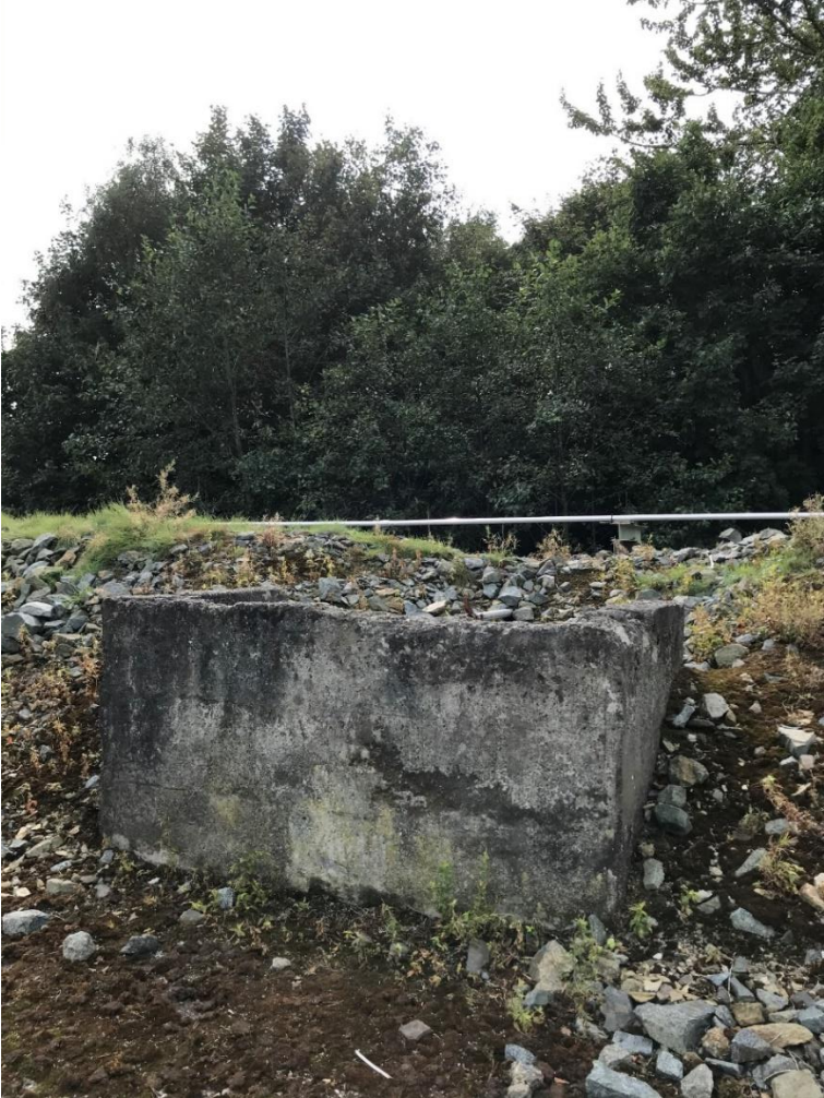
Location of possible erosion or changes in embankment level associated with historic infrastructure on southern embankment.
